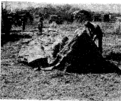
These members of the 586th FLOAT Bridge Co. had the task of inflating the rafts which supported the road surface of the bridge. Over 50 such rafts were used to keep the emergency bridge floating. (U.S. Army Photo)
