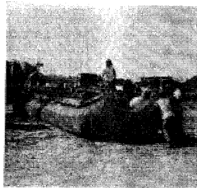
It takes a lot of hard work on the shore just to get the section of the bridge ready to put into the water as these engineers demonstrate. These engineers are working to secure the super structure to the rafts. (U.S. Army Photo)
