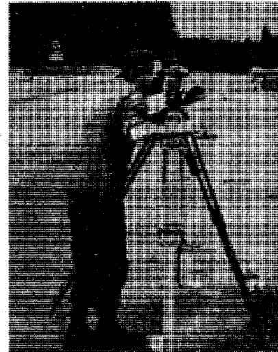
Without a surveyor, constructing a roadway would be time-consuming, if not impossible. SP4 Hardwich, of the 43rd Engr Bn, is one of the unsung heroes who makes the any road construction job easier. (Photo by Gary Cathcart)
